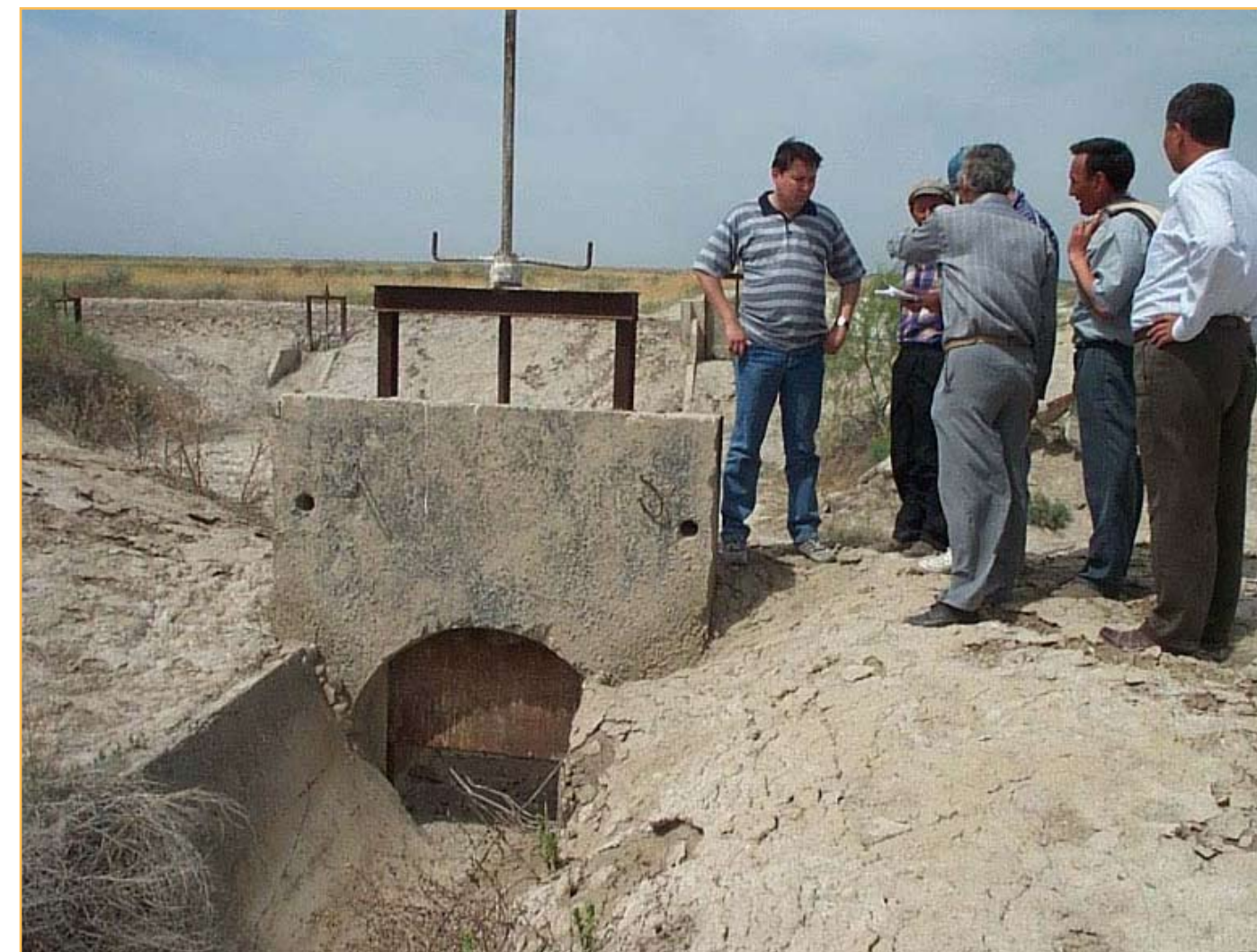
Inspecting a damaged irrigation systems in Kazakhstan
