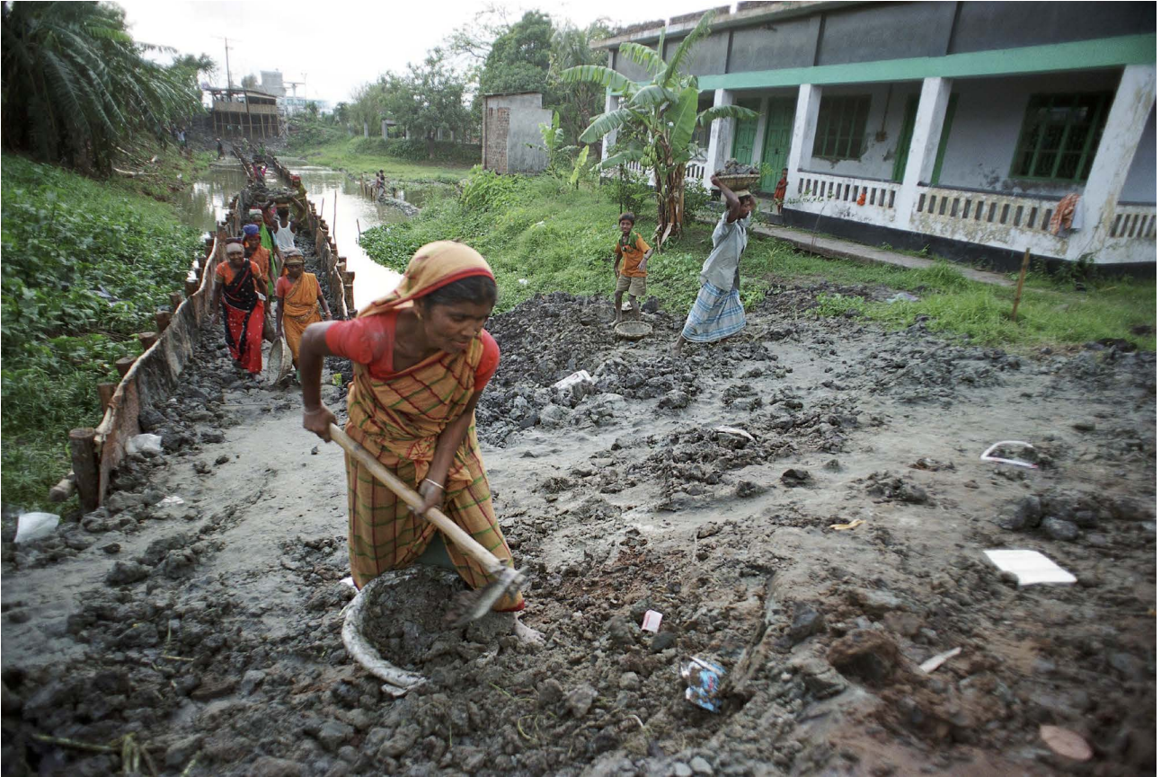
Bangladesh, preparing to build a road. Photo credit: Scott Wallace/World Bank via Flickr, CC BY-NC-ND 2.0
