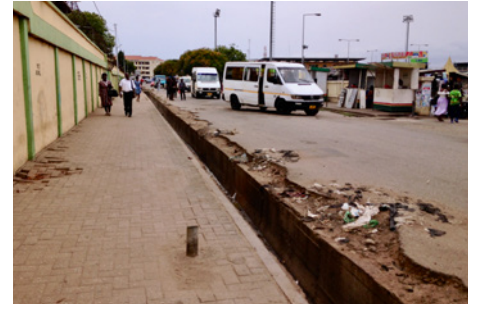
Uncovered drains along many streets
