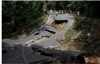
A highway in Getafe, Bohol damaged by the earthquake - Reuters
