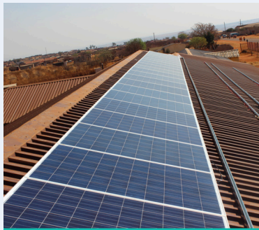
Solar panels are installed on a community centre in Steve Tshwere Local Municipality, South Africa, during phase I of the Urban-LEDS project.
