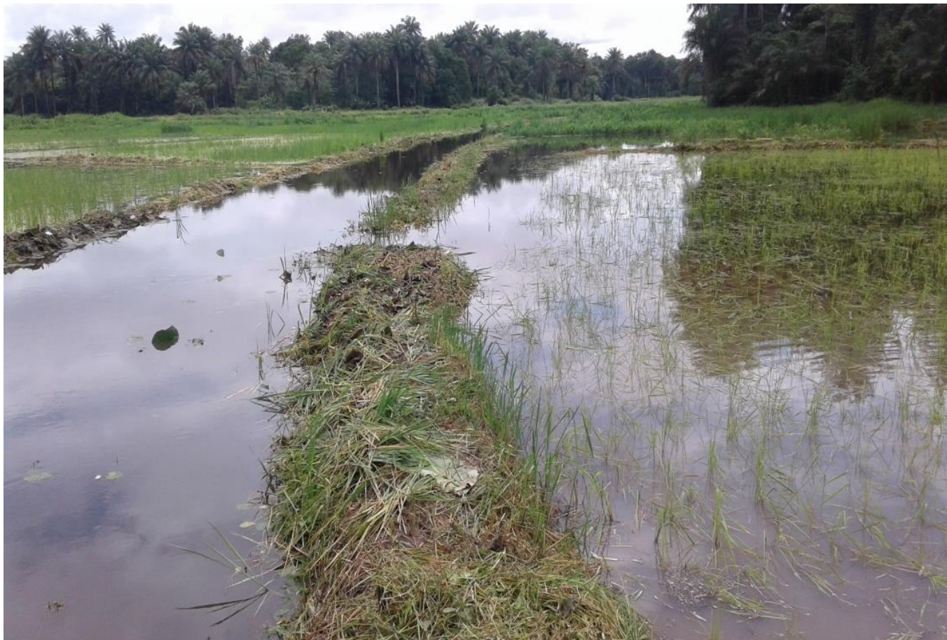
Figure 1: Lowland irrigation structure damaged by heavy rainfall, Roline, Maforki chiefdom, Port Loko district (Sulaiman Coker, WFP)
