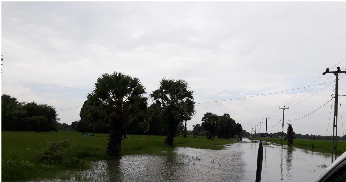
Submerged Road in Puliampokkanai in Kilinochchi on 26 December (Photo Credit WFP)
